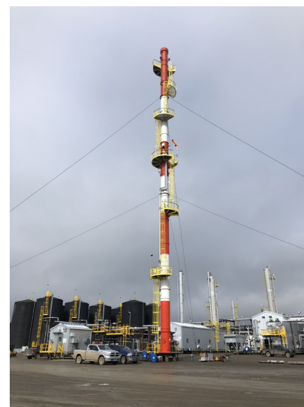
Exhibit 5: Questor Q5000 with 160ft Stack; Acid Gas Processing in British Columbia
