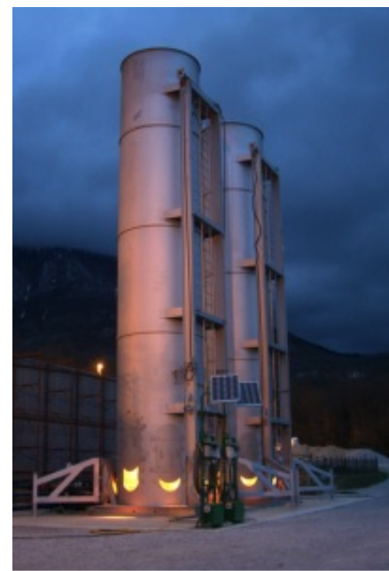
Exhibit 4: Questor Q3000 Combustor Operating During Flowback
